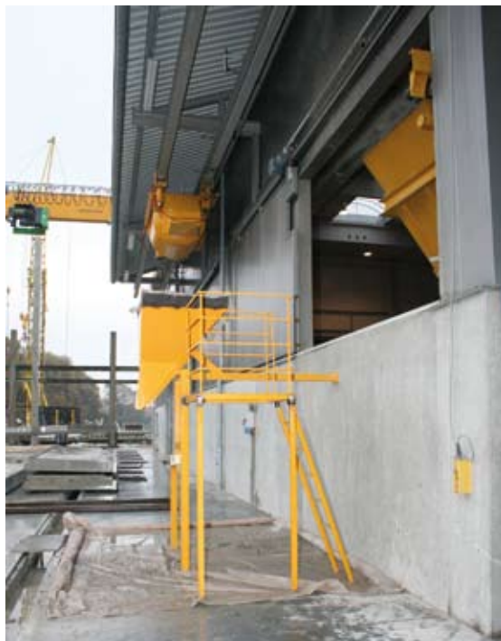
Fig. 1 The silo is fed via the outside bucket conveyor supplied by company WMW.
