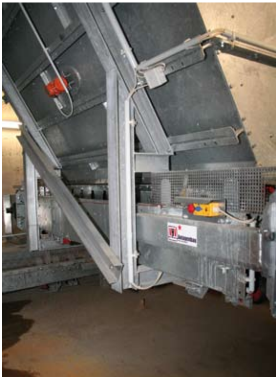
Fig. 6 Inside the feeding bunker where the aggregates are transported to the double belt conveyor by the transverse conveyor belt: material bunker for 20 m 3 of gravel with discharge conveyor.
