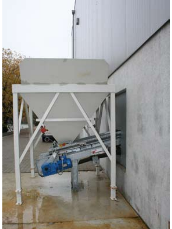
Fig. 5 The production hopper for special aggregates: big bag discharge through outside hoppers and dosing conveyor possible.
