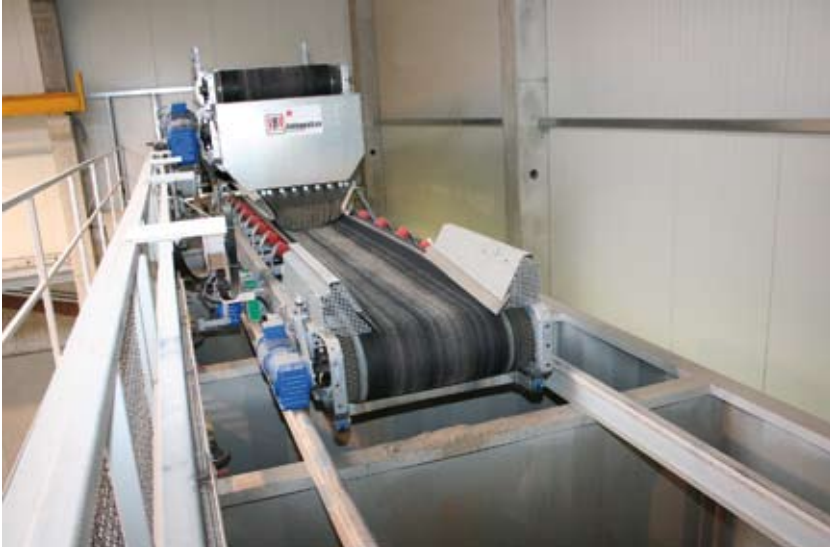
Fig. 8 In this way, the raw materials are carried from the double belt conveyor into the single silos. Abb. 8 So gelangen die Rohstoffe vom Doppelgurtförderer in die einzelnen Silos.
