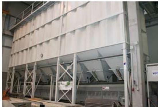
Fig. 3 The row-type silo plant with dosing flaps and weighing conveyor at the head end of the production building.
