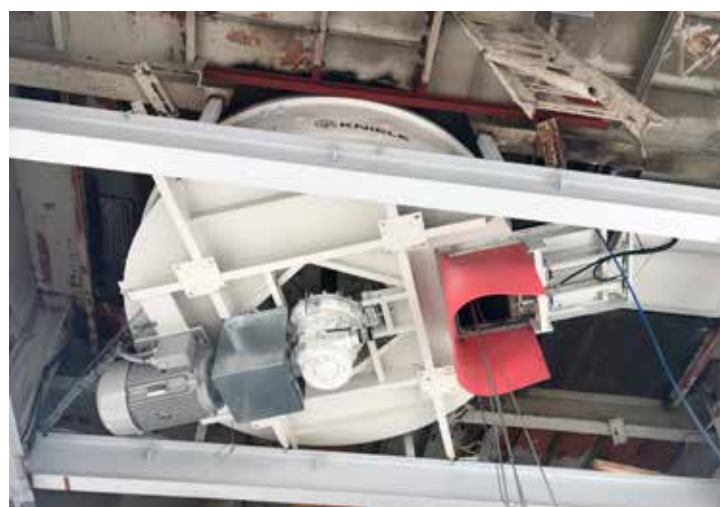
Following disassembly of the two existing mixers, the new ring-pan intensive mixer was installed in the supporting scaffolding
